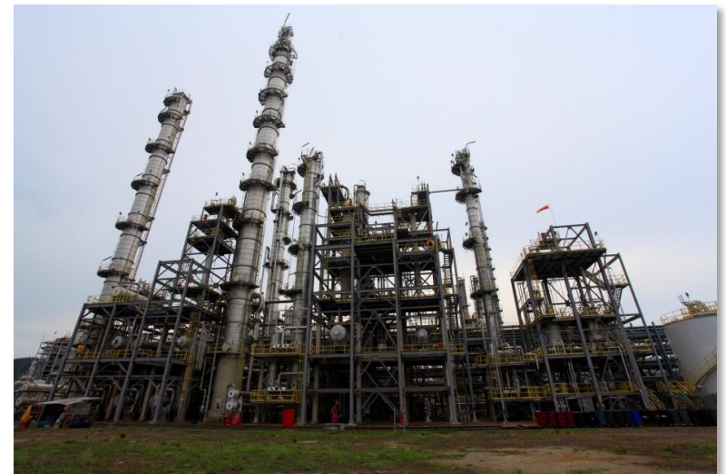
Existing BD plant in Cilegon with capacity 100 KTA.
